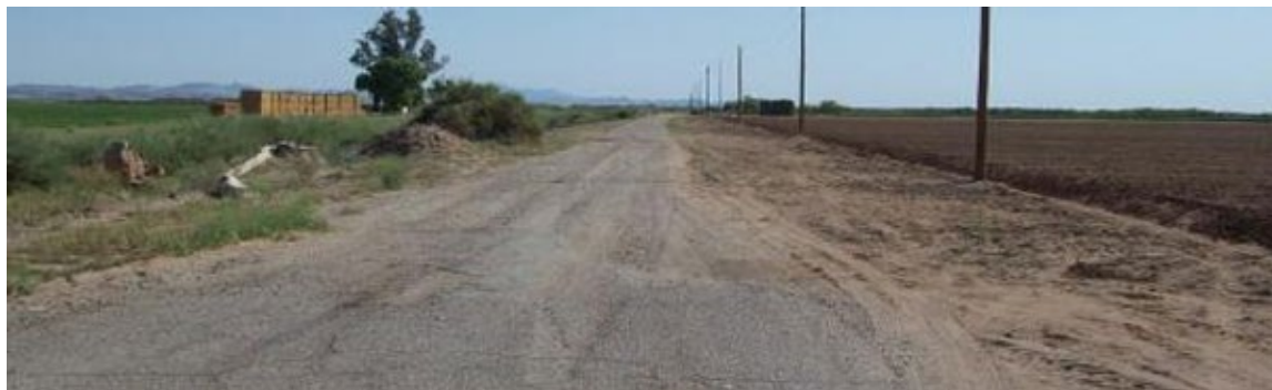
Example of a roadway with very poor pavement condition
