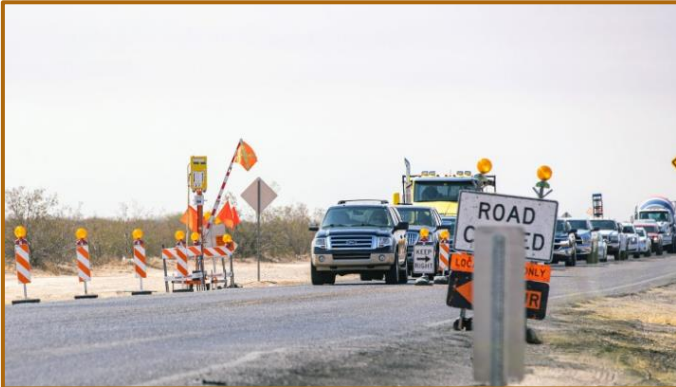
SPECIAL TO INDEPENDENT NEWSMEDIA / ARIANNA GRAINEY Construction lasted year along Hunt Highway in Pinal County near Florence
